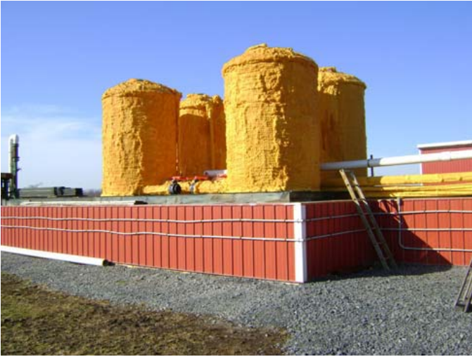
Figure 2. Hydrogen Sulfide (H 2 S) Scrubbers
