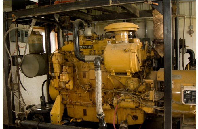
Figure 3. Caterpillar ® SGE setup in operation
